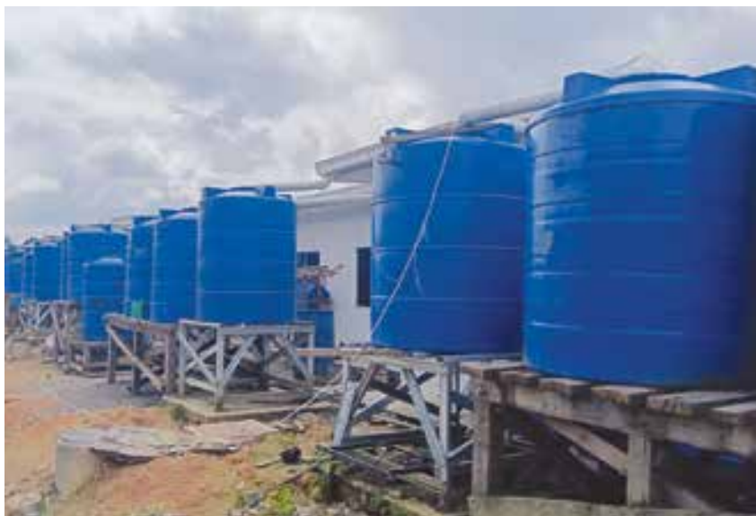
Rain water harvesting tanks
