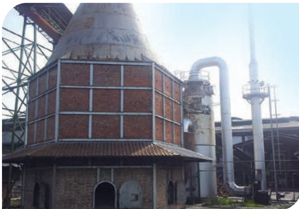
Incinerator at Mukah Palm Oil Mill
